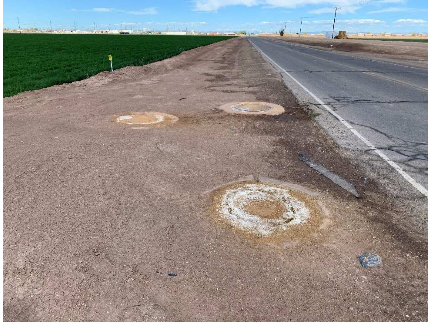
Manhole #359 (located in foreground) and two unnumbered manholes to be removed. View north on the western side of Clark Road.
