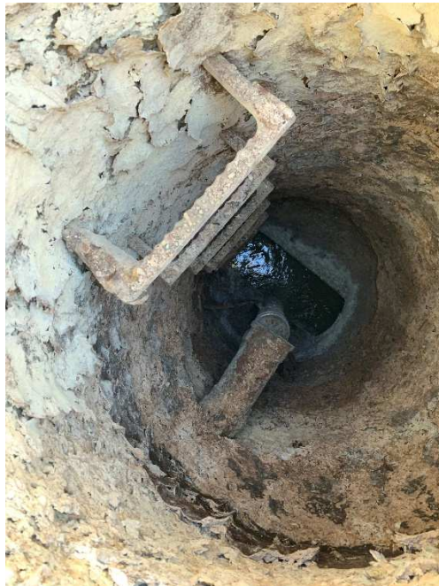
View north within MH No. 1102 (stairs to be cut/removed)
